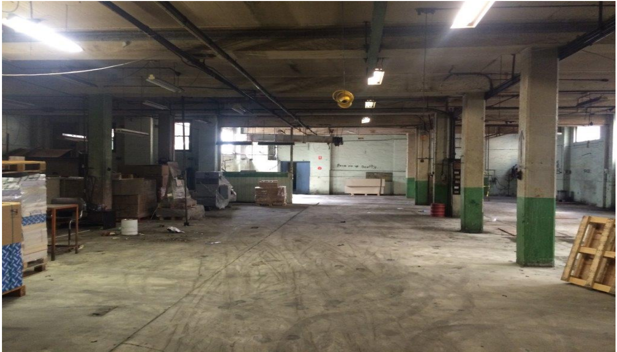
Photograph 1: Site 3, 305-309 Trafalgar Street, warehouse interior, oil staining on concrete surfaces, metal and wood scrap materials noted throughout.
