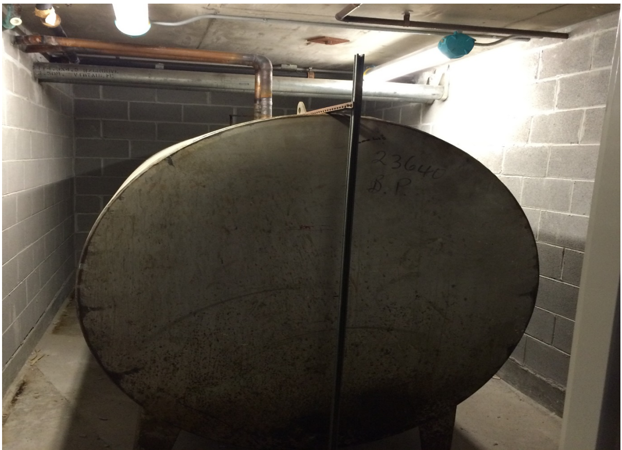
Photograph 6: Site 1, Underground car park, Diesel above ground storage tank.
