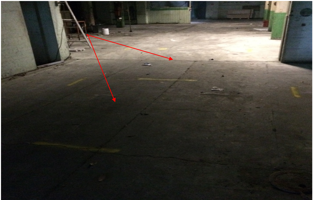
Photograph 4: Site 3, 305-309 Underground Storage Tanks identified adjacent to roller door.
