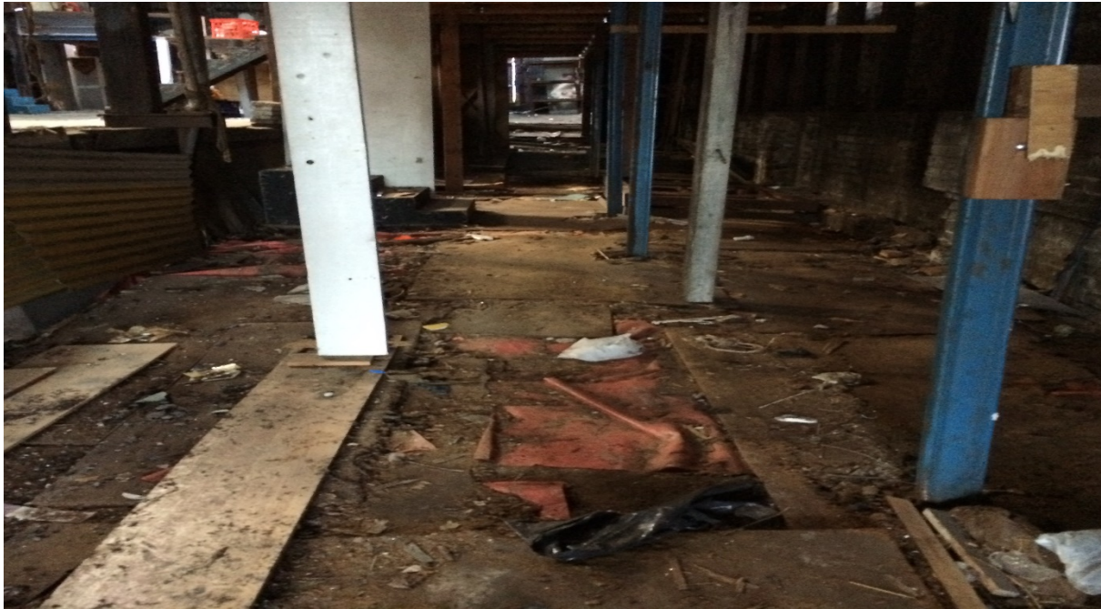
Photograph 5: Site 3, 301-303 Trafalgar Street, plastic wood and metal scrap material throughout, no hardstand cover noted throughout the footprint of the warehouse.
